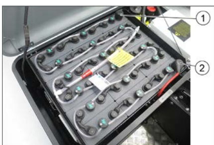
Battery terminals - travel direction left
